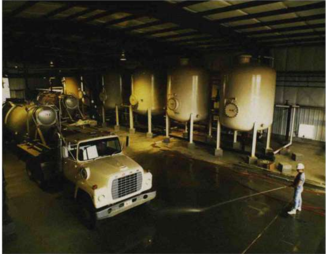
Figure 15 Satellite Ion Exchange Columns with Resin Trailer –
